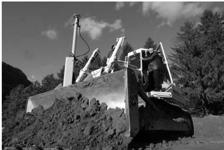
Fig. 6: The construction machine is equipped with a Leica dozer system, which determines the 3D position of the blade in real time to the nearest centimetre. The driver of the machine receives all guidance details directly from the system.
